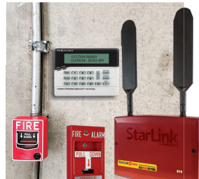
SECURITY & FIRE ALARMS & REPORTING
